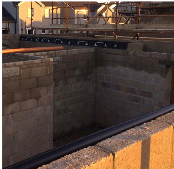
Figure 1: Aerstad System installed on site
